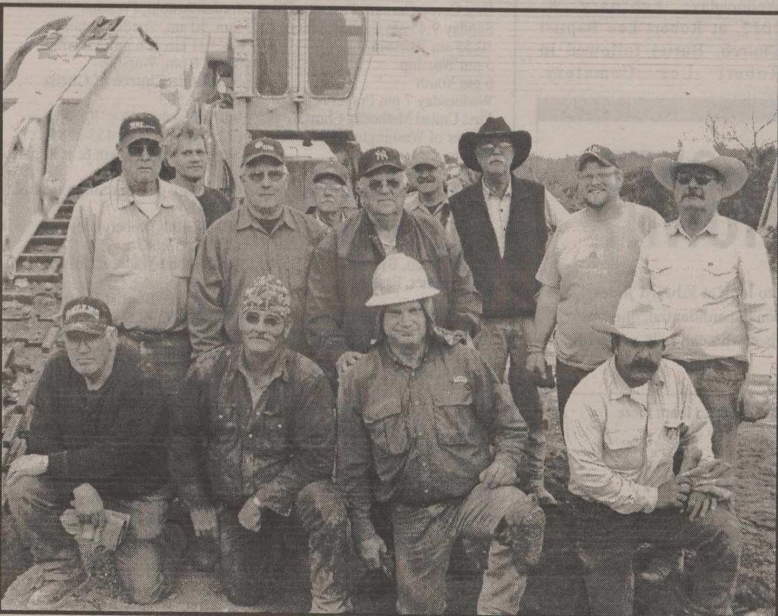
Robert Lee Pipeline! This group of volunteers worked late on Thursday, February 2, 2012, to complete the 4.5 mile portion of the waterline to Bronte. The pipeline contractor will be responsible for the remaining 7.5 miles to the treatment facility at Bronte. The volunteers will finish up the project this week by tying the pipeline in to Robert Lee's treatment plant.
