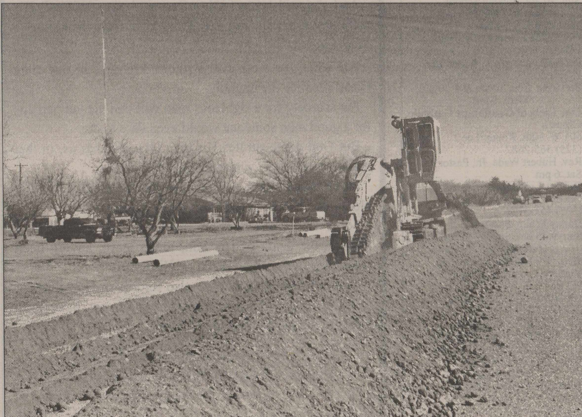
It's Begun! The trench for the water pipeline is under construction. Digging began Tuesday, with the machine and its operator being donated by Vermeer.
