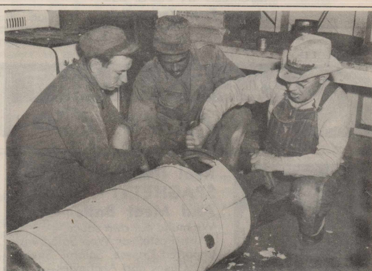
REPAIRING A HOT WATER booster heater may not be as easy as it looks. B. E. Dunsworth, civilian worker (right) explains the functions of the heater to Pvt. Herman Murman and PFC Hector Osie (center).
