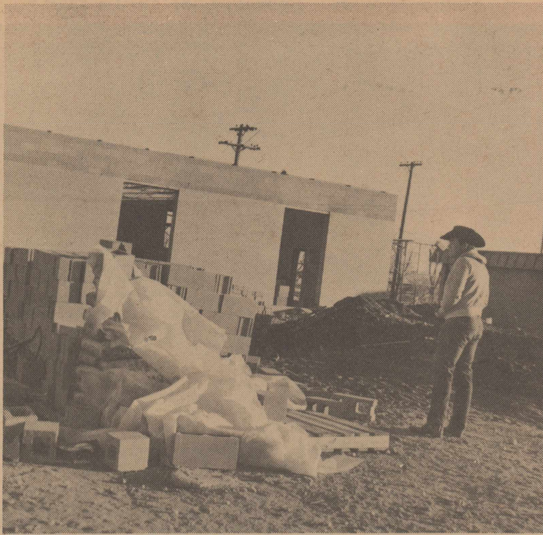
The Raymond E. Buhman Construction Company is completing the new bus barn being built adjacent to the M. S. Doss Scout Center. Jack Ramsey, construction company foreman, is looking on.
