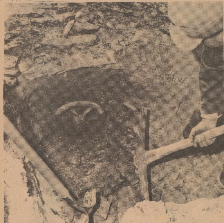
If you wonder why the City continues to dig up the middle of the streets this is reason enough. Here's a 6" valve below street level that had a 4"x8" opening to operate it. Just north was a fire hydrant in the street that had to be moved for the new paving. City employees are shown digging out the valve so they can cut off a 6" main so that a fire hydrant can be moved so new pavement can be put down at the corner of S.W. Ave. B. and 3rd Street. (Real planning, huh?)
