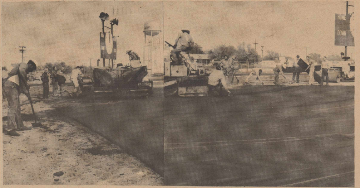
Crews are putting the finishing touches on the new all weather track at the football field. Equipment shown here is presently laying the topping for the high jump runway. (Everyone is asked to help take care of the new surfacing.)
