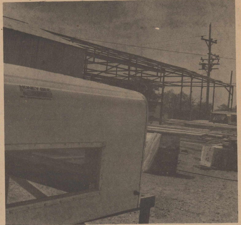
Honey Bee Campers is building a new addition onto their building in the 800 block of South Main. It was formerly known as Seminole Mill Works. The business has been in operation for three months. Isabel Alaniz is the owner. The firm builds covers for pickups, campers that fit in the back of a trailer and small vacation trailers.
