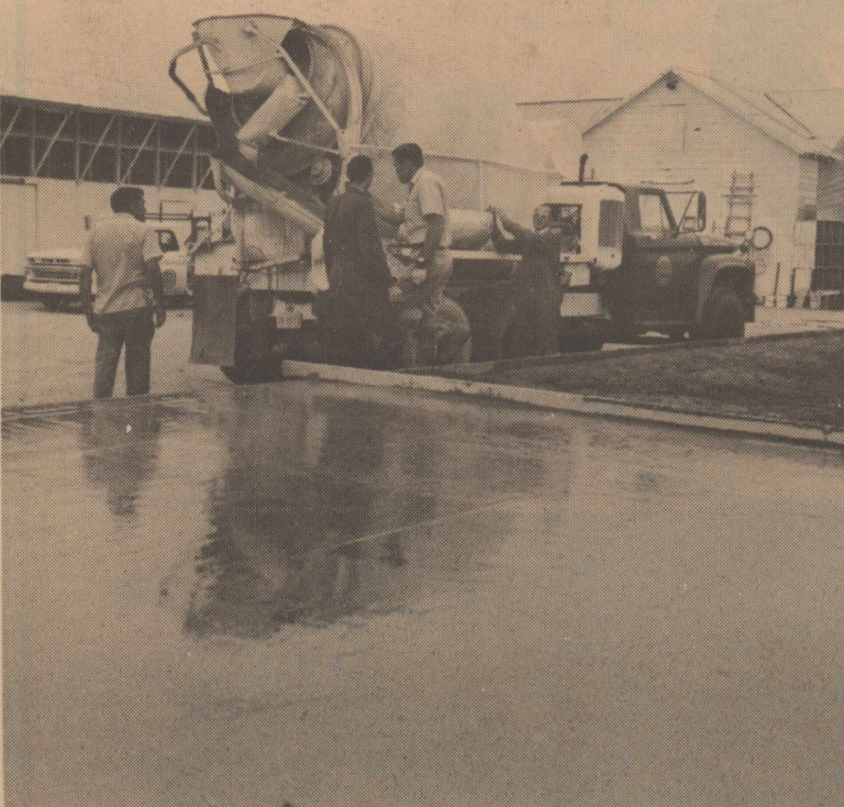
Forrest Lumber Company pours the floor for their new building. Shown are Howard Deen, Jerry Shipley and Henry Hitch.
