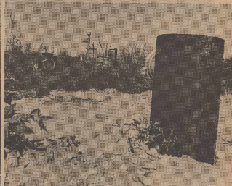
Things are BIG in Texas and Gaines County. These underground risers measure 16" and have valve take-offs of 8". That's a gas meter between the two risers.
