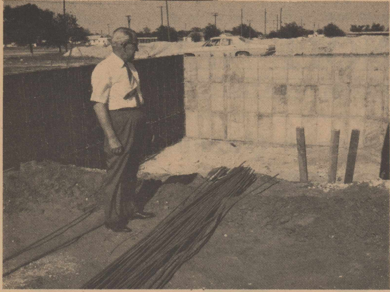
Doyle Hankins, executive officer of the Seminole State Bank, views the excavation at the bank's new building site. He states that they hope to be in the new structure by December 1, 1969.
