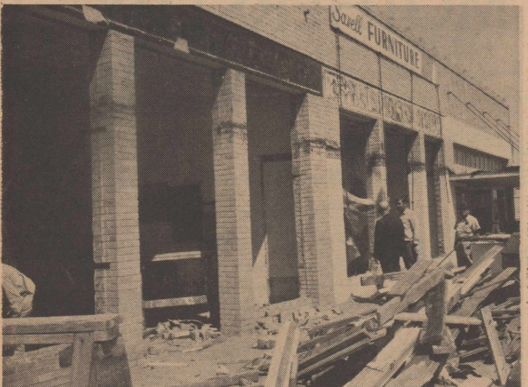
Hurray for Jack Jordan and Jordan Furniture Company, George Abe and Glen Weiser (owners of the buildings) for reworking the building fronts on the west side of the square. Reeves Cothes was reported as saying the buildings were built approximately fifty years ago. THEY NEEDED A FACE LIFTING!
