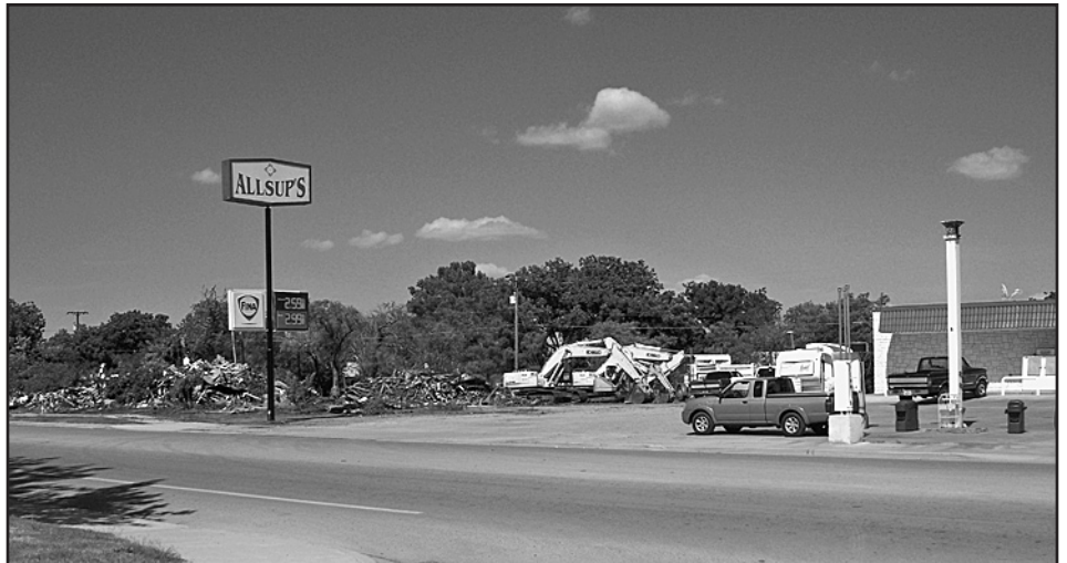
EXPANSION PROJECT —Allsup's in Haskell, located at 1000 N. Ave. E, has bought adjoining properties and is expanding their business to include more pumps and a larger parking lot.
