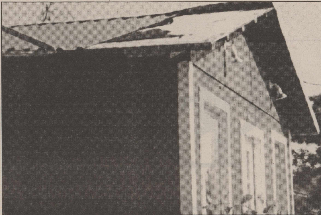
Storm Damage! Robert Lee residents will have to put their pizza cravings on hold awhile longer after Vincent's Pizza Place was damaged during a recent storm. Vincent Puthoff was scheduled to open the new business shortly, but now will have to complete repairs before he can open his doors to the public.
