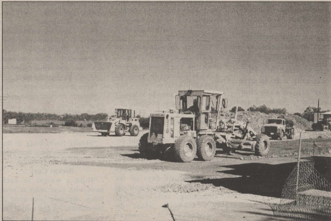
Construction Begins! Construction began recently on Bronte Independent School District's new gymnasium. The newest of the three gyms will be located behind the school. The gym is not expected to be completed for use this school year.
