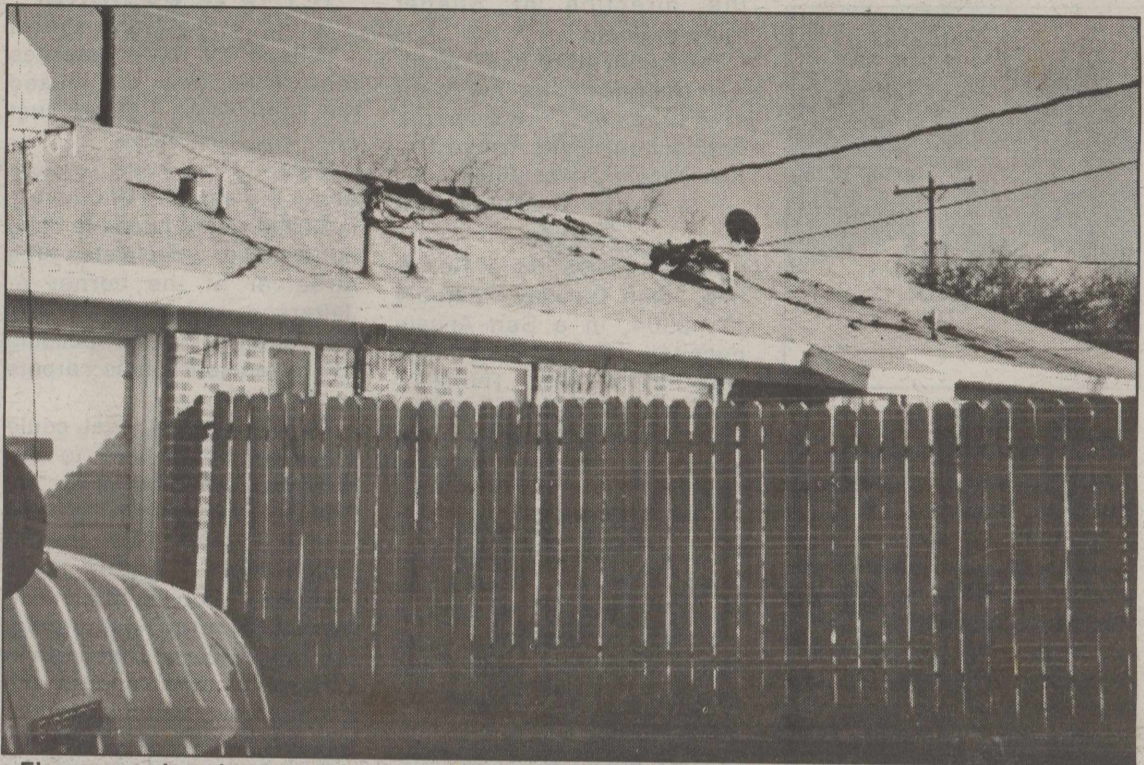
Fire caused major structural damage to the home of Gary and Annette Acker Tuesday afternoon, February 17, 2004. The fire began in the attic and was extinguished by members of the Bronte Volunteer Fire Department. The home is located at 402 S. Washington in Bronte. A fund has been established for the Acker family at First National Bank in Bronte.
