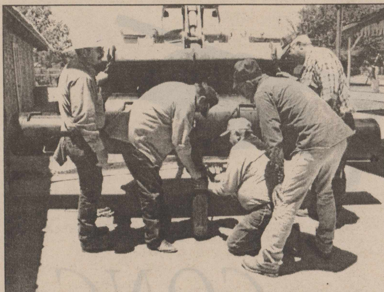
Volunteers work to install the new barbecue pit at the County Park in Robert Lee. The new 13 foot pit, a West Coke County Community Development project, will hold up to 15 briskets at one time. Shown are (from left) Tim Millican, Gene Montgomery, John Carver, Tommy Shook, and Gaylon Pitcock.
