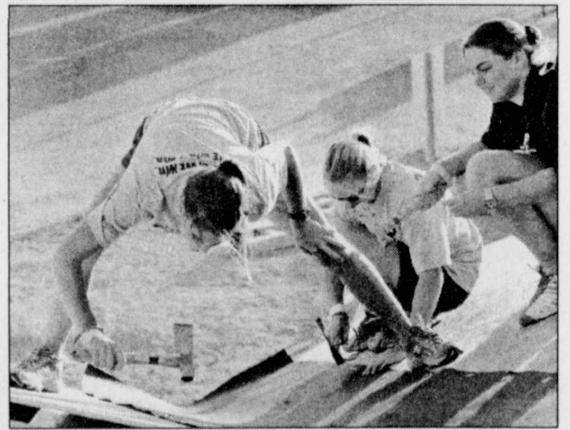
TOP: LAKANN WAGLEY, a freshman tennis player, moves a roll of roofing felt up a ladder. ABOVE: Wagley and teammates nail down roofing felt on the house the team helped build as part of Habitat for Humanity.
