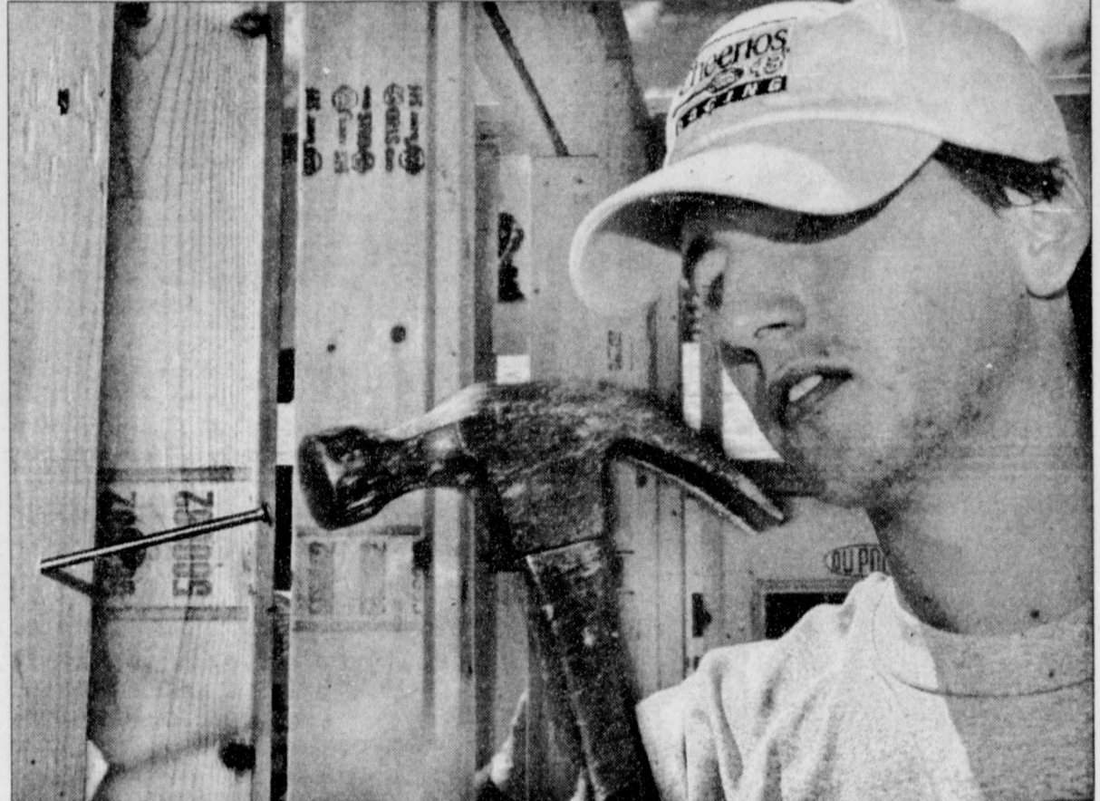
TECH HABITAT FOR Humanity member Q.T. Felton, a sophomore mechanical engineering major from Houston, helps put up the walls on a Habitat house on the 2200 block of Duke Street during the Habitat for Humanity Blitz Build on Saturday afternoon.
