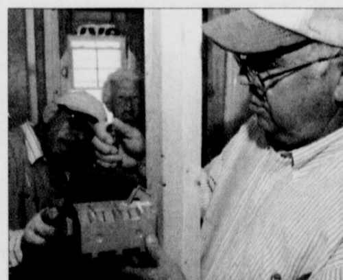
JAMIE TOMAS AGUILAR/Staff Photographer LEFT TO RIGHT, Mohammad Shayib, a systems analyst for the graduate school, Lubbock resident Ruthie Dean, and Associate Dean of Civil Engineering John Borelli work together to install the electrical wiring inside of the "Abraham House."
