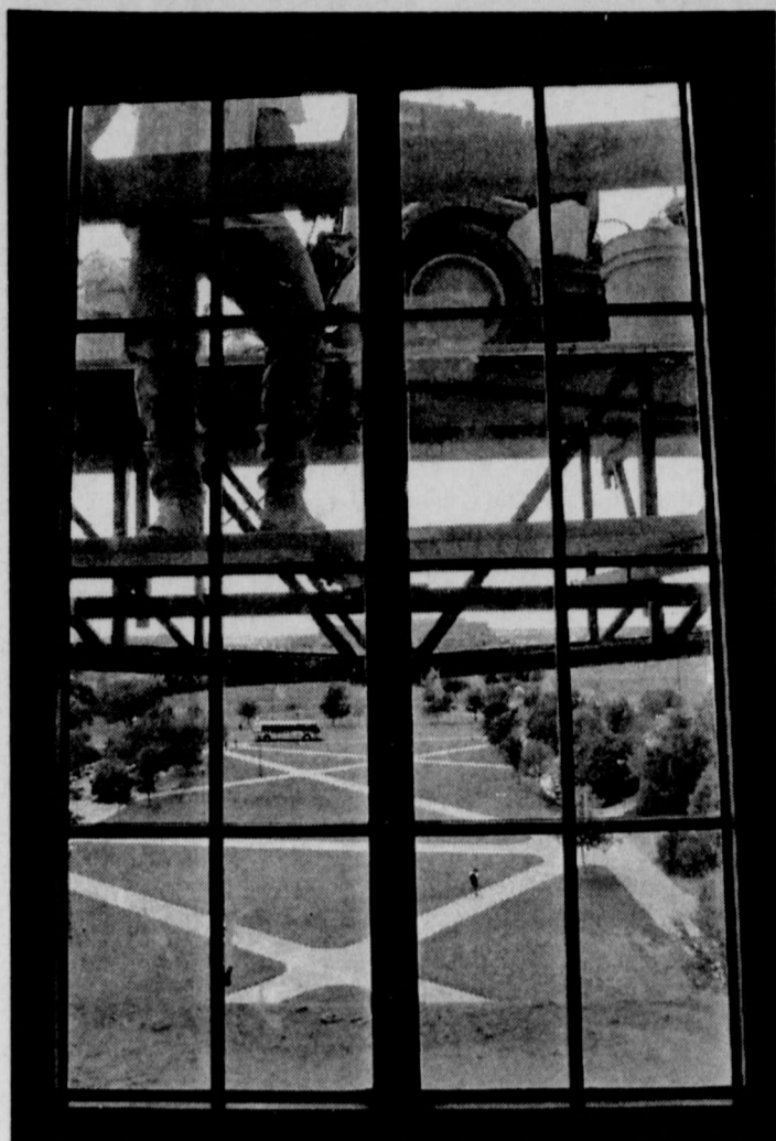
GREG KRELLER/Staff Photographer A CONSTRUCTION WORKER is seen through the window of the English building Tuesday afternoon. Finishing touches on the building are still in progress. Faculty and staff began moving into the new building in July.
