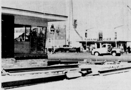
PARADE OF PROGRESS--New additions to buildings in Muleshoe are currently underway in the area. Shown here is an awning being constructed at the new Corral Drive Restaurant on West American Blvd. It was opened last week by Roy Dyer.
