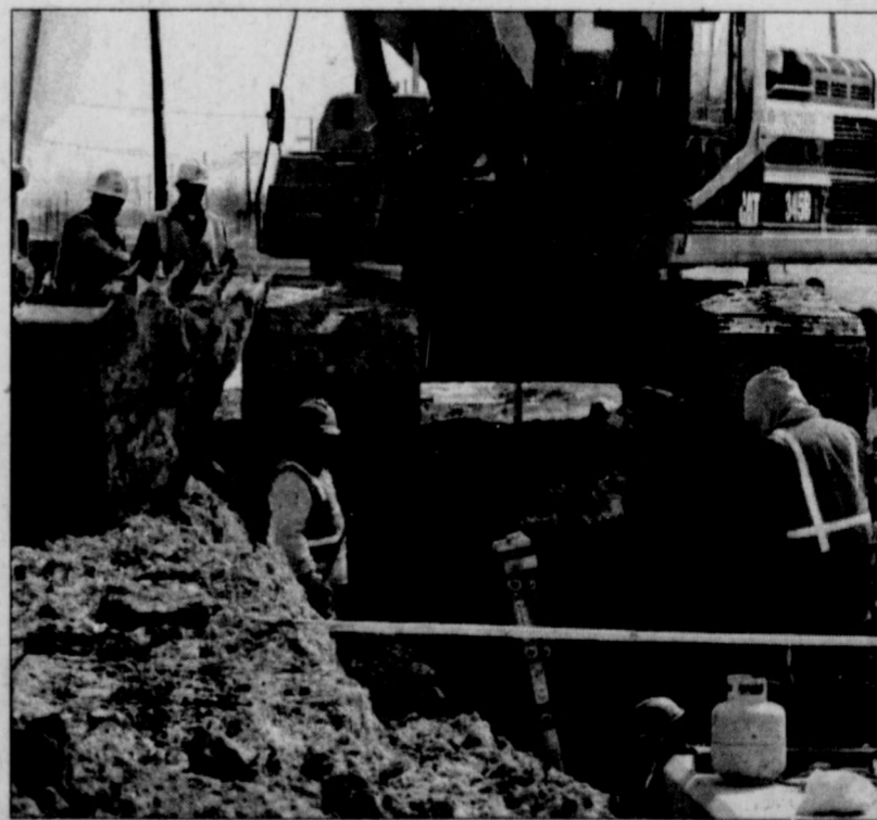
DAVID JOHNSON/Staff Photographer WORKERS INSTALL A pipeline at the corner of Milwaukee Street and 19th Street.
