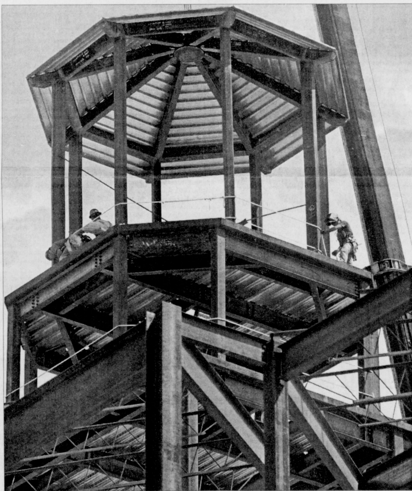
WELDERS AT THE English/Philosophy/Education Complex fasten the top of the tower above the English/Philosophy building Tuesday afternoon as they continue to work on the project which has lasted more than two years. Texas Tech officials will hold a topping off ceremony at 3:30 p.m. Thursday to honor the project's progress.
