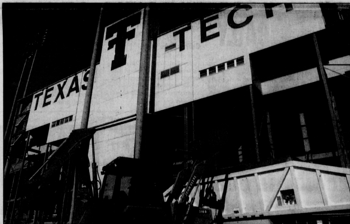
A worker disposes of debris from the former segment of Red Raider Avenue west of Jones SBC Stadium.
