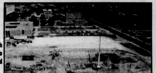
▲ Construction of the both the north and south basements are scheduled to be completed within two weeks. The total cost for the English/Philosophy and Education Complex is estimated at $45 million.
