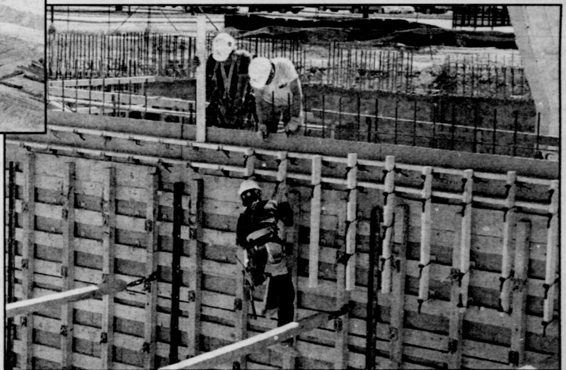
▲ Workers build form work for the basement walls, which will be filled with concrete during the next two weeks.
