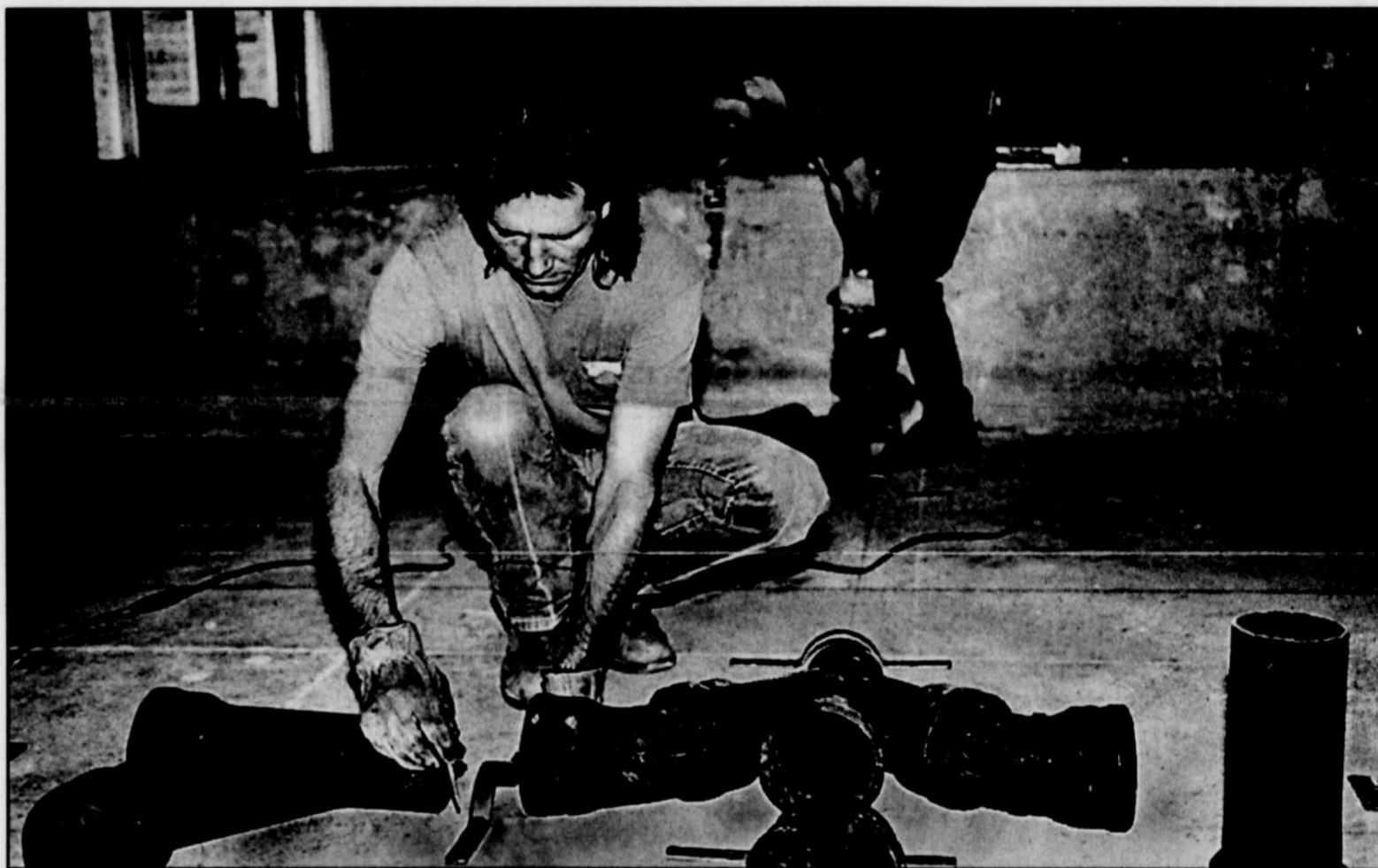
Plumbers Sammy Smith and Chad Price begin installation of pipes for bathrooms in West Hall. The $6-million project is slated to be finished in April 2001 and will include a new visitor's center and asbestos abatement.
