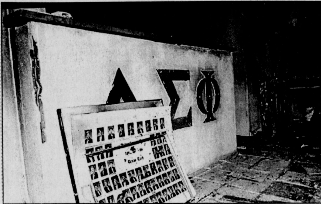
Damaged: Only charred remains are left at the Delta Sigma Phi fraternity lodge, 2407 Main St., Monday after an early morning fire. Fire Marshal Marlon Hamilton said the cause of the fire is arson and that damages are estimated at about $32,000. He said arson and vandalism were probably an attack at fraternities in general, not just Delta Sigma Phi.
