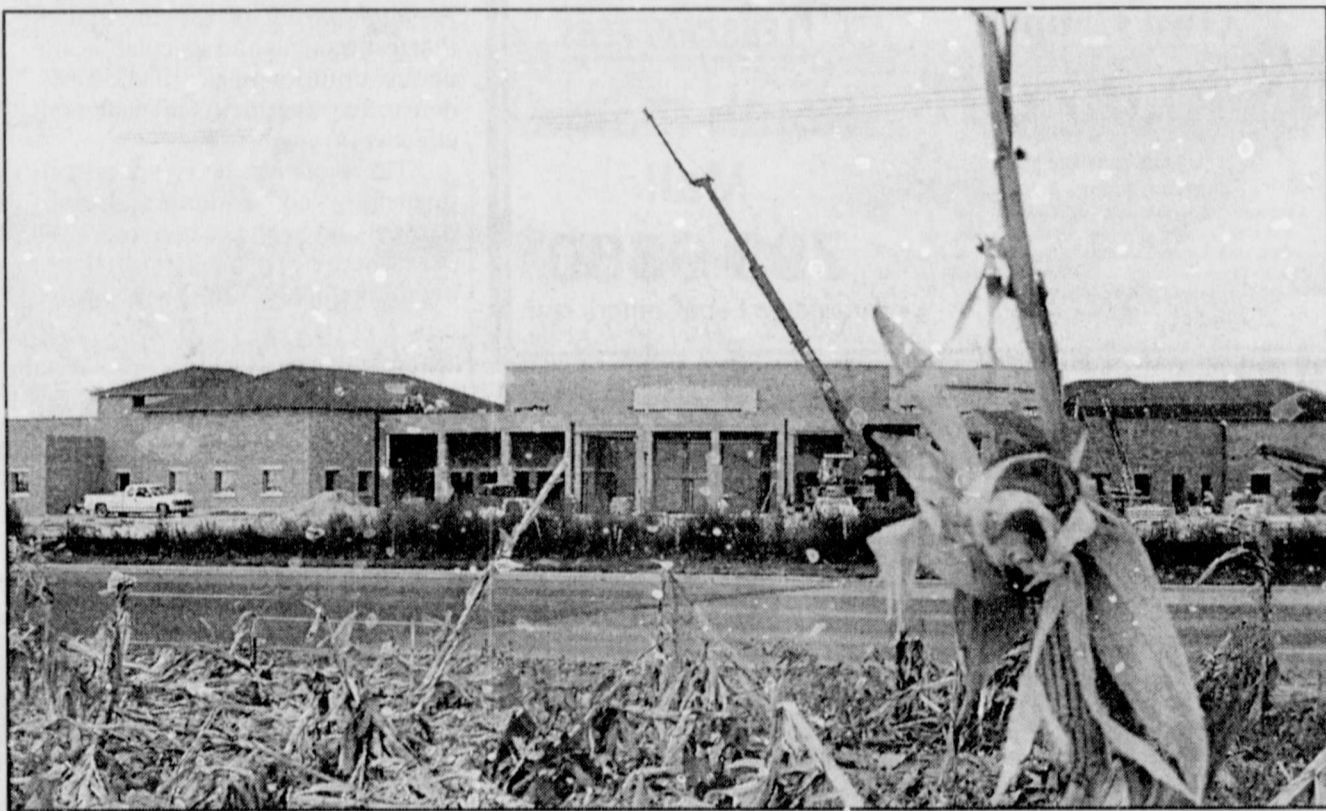
Halfway There: Construction for the USDA's Plant Stress and Water Conservation Laboratory at Texas Tech is almost complete. The lab, located at Fourth Street and Memphis Avenue, is expected to be finished Jan. 21.
