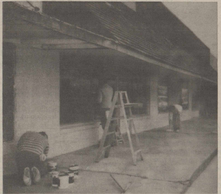
West Coke County Community Development made a start last Saturday on its Downtown Project. Billy Kelly and Gary Williams paint in the foreground while Noel Tinkler works down the sidewalk a ways. Another workday or two will be set soon.
