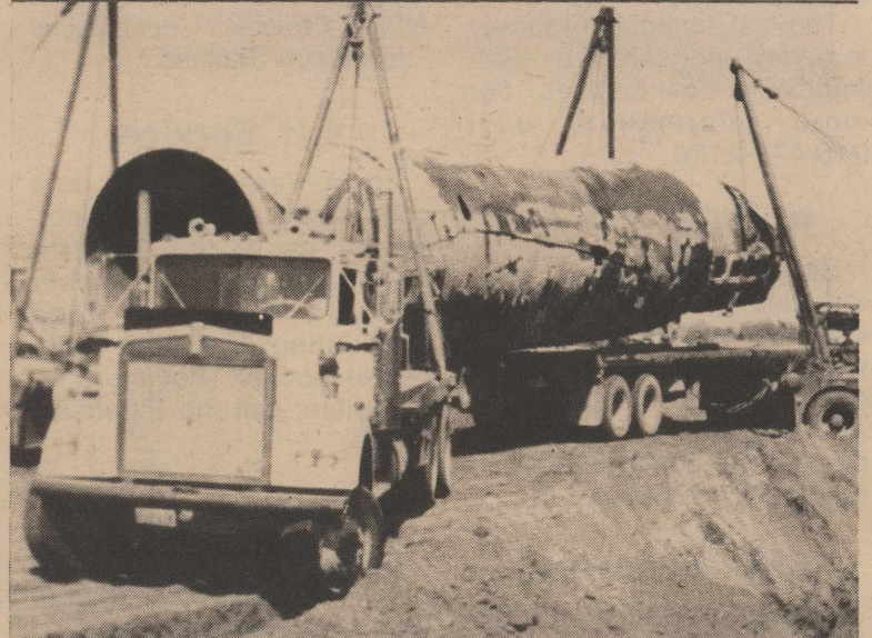
Two oilfield tandem trucks jockey a 10' diameter "tinhorn" into place to permanently repair Exxon Road off West Hwy 208 on Rough Creek near Lake Spence.
