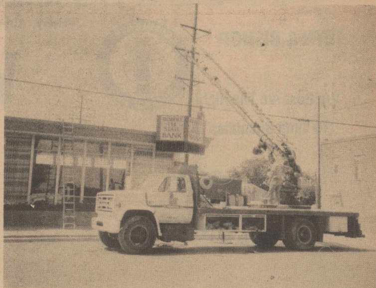
WORKMEN MAKE THE final adjustments on the new sign which will grace the front of the Robert Lee State Bank. According to Willis Wayne Smith, bank spokesman, the time and temperature functions of the sign will be in operation soon, just in time for the triple digit summer weather we have experienced recently.
