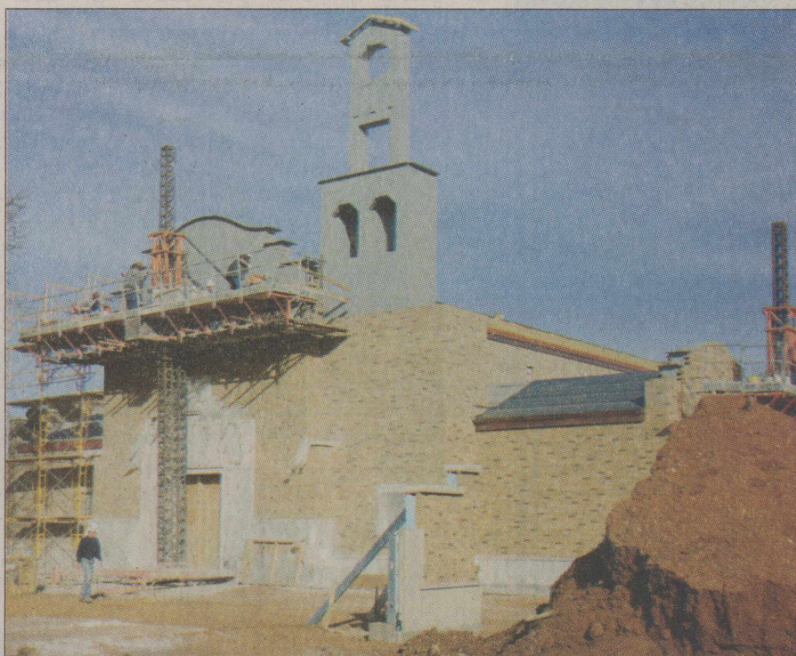
PHOTOS BY EMILY DE SANTOS /The Daily Toreador TOP: CONSTRUCTION WORKERS continue to make progress on the school's new Boston Ave. Residence Hall and Dining Facility on Wednesday. ABOVE: Workers continue construction on the Kent R. Hance Chapel.
