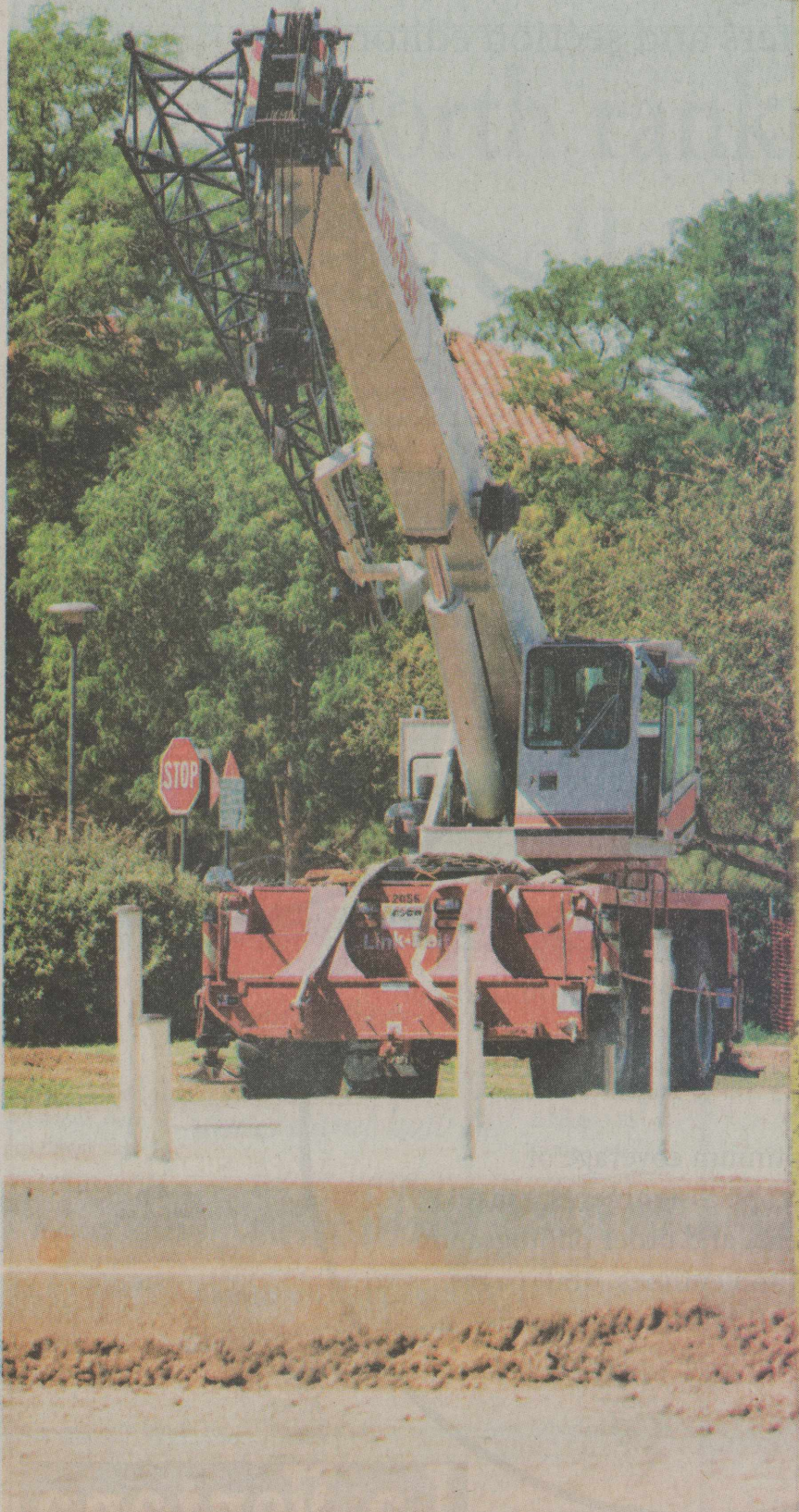
A CRANE IS on sight Tuesday near the foundation of the Kent Hance Chapel which is being built near the Merket Alumni Center.
