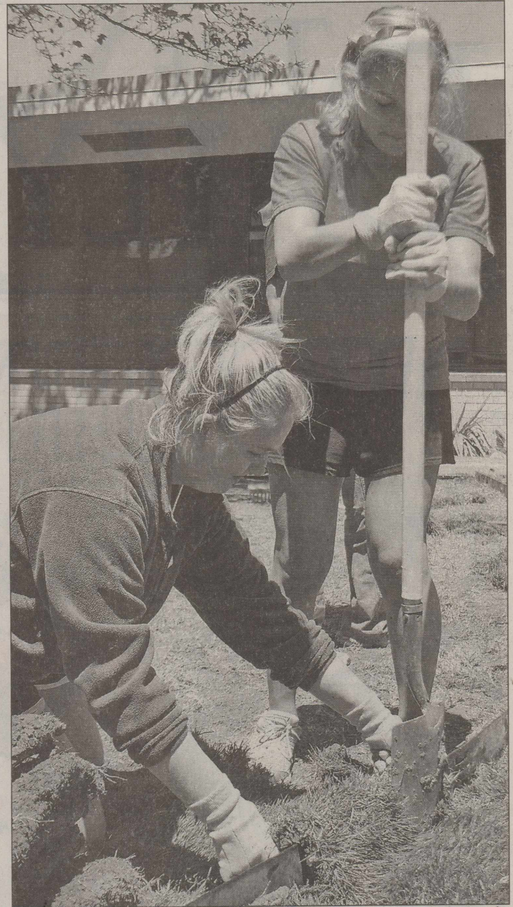
PHOTO BY RIANNON ROWLEY/The Daily Toreador LINDSAY PARIS, LEFT, a junior early childhood education major from Plano, and Kendall Walters, a sophomore early childhood education major from Katy, work with project G.R.I.P. on completely renovating Jackson Elementary School's courtyard Saturday.
