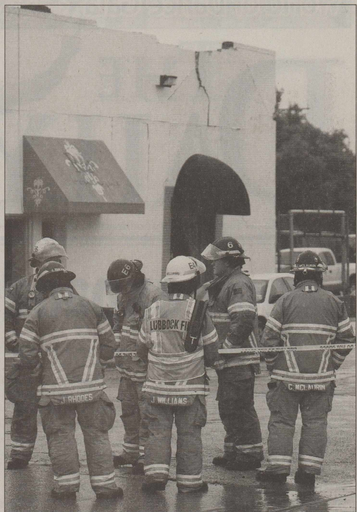
PHOTO BY BRAD TOLLEFSON/The Daily Toreador MEMBERS OF LUBBOCK Fire Department assess the damage caused by rainwater collection to the roof of the Little Panda Restaurant at University and Broadway.
