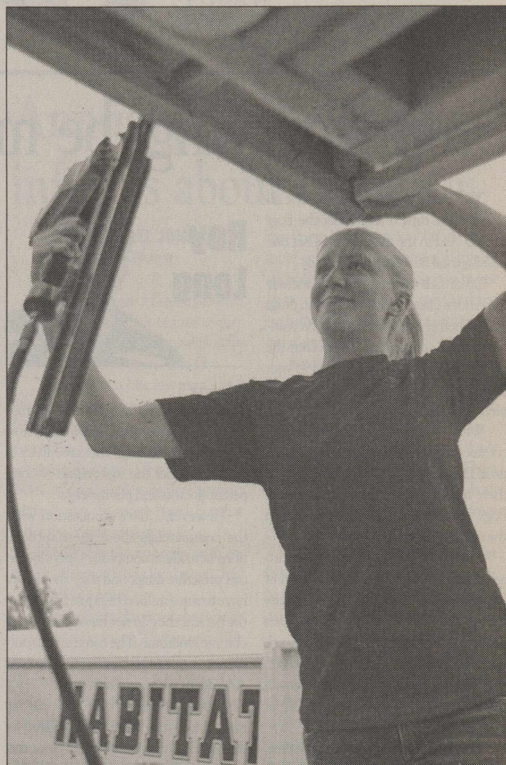
PHOTO BY BRAD TOLLEFSON/The Daily Toreador KACY CHANDLER, A freshman animal science major from Hale Center, nails up a support board for roofline on the outside of the house.
