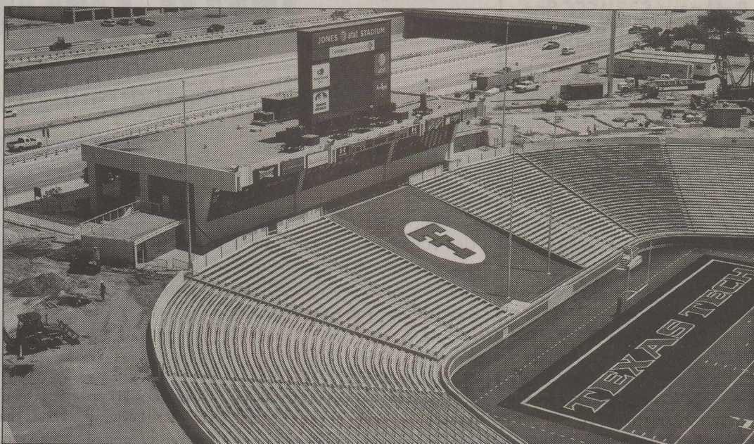
PHOTO BY KEN MUIR/The Daily Toreador CONSTRUCTION ON THE north side of Jones AT&T Stadium is underway and is expected to be usable by the Oct. 24 football game against Texas A&M University. The expansion will add an extra 6,000 seats to the stadium.
