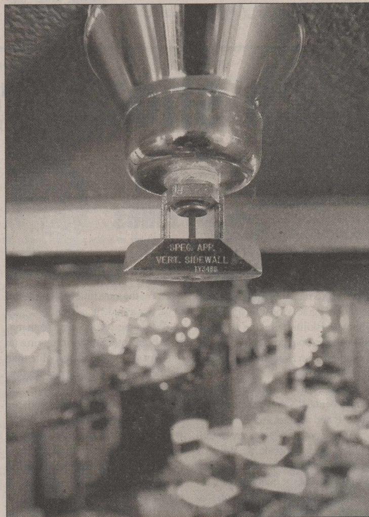
PHOTO BY KARL ANDERSON/The Daily Toreador THE SPRINKLER SYSTEM in the residence halls sprays 20 gallons to 30 gallons of water per minute, preventing the spread of fires. The sprinklers will set off at temperatures at or above 145 degrees or if they are tampered with.
