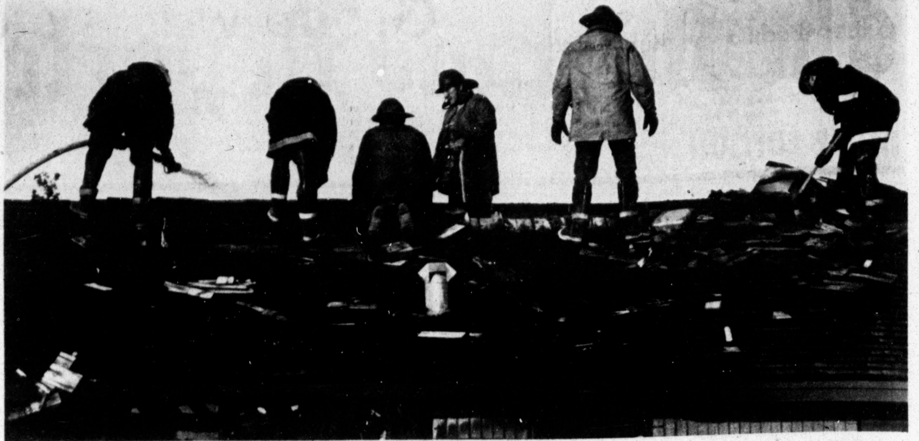
Half a dozen Midland firemen rip out shingles and water down the roof of a residence under construction at 2608 Castleford Ave. about 6:30 p.m. Wednesday. An overheated air conditioning unit is suspected in the fire, which caused extensive damage to the vacant northwest Midland house. Harvey Langston Realtors had a contract signed on the new home, but had not closed with the buyers. Firemen worked for about 1 1/2 hours to extinguish the blaze. (Staff Photo by Bruce Parntain)
