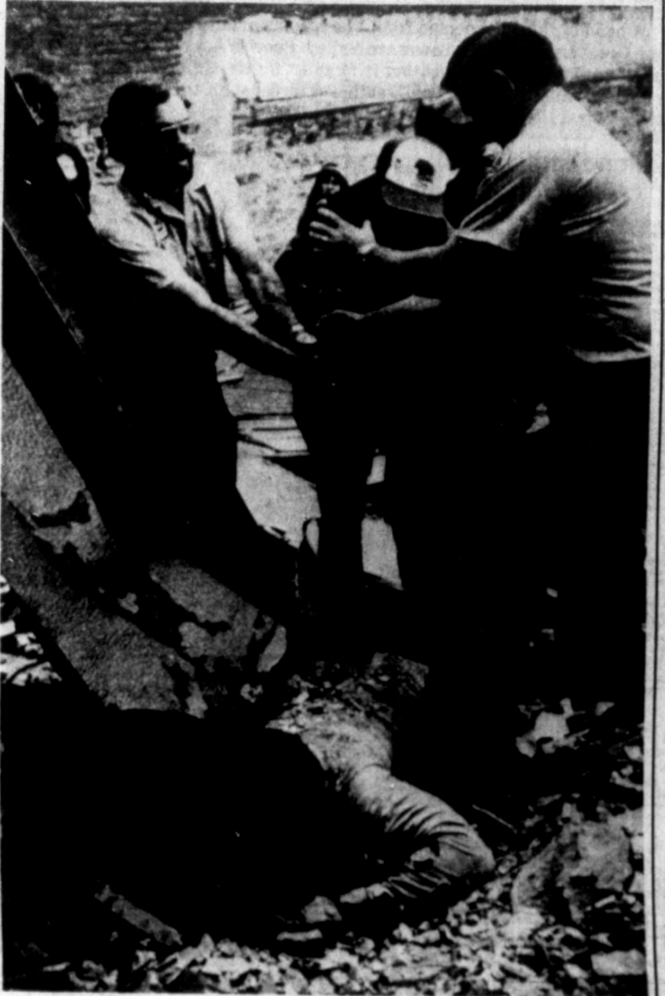
A demolition worker, Ronnie Jones, is freed by rescue workers after being pinned by a steel beam when the second floor of a building in which he was working in Ottumwa, Iowa, collapsed. Three co-workers, including Jones' father, died in the mishap, and emergency workers said Jones' back and legs were broken. (AP Laserphoto)
