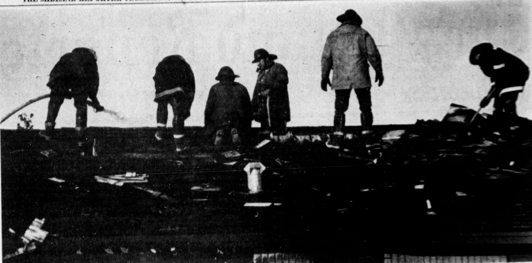
Half a dozen Midland firemen rip out shingles and water down the roof of a residence under construction at 2608 Castleford Ave. about 6:30 p.m. Wednesday. An overheated air conditioning unit is suspected in the fire, which caused extensive damage to the vacant northwest Midland house. Harvey Langston Realtors had a contract signed on the new home, but had not closed with the buyers. Firemen worked for about 1 1/2 hours to extinguish the blaze. (Staff Photo by Bruce Par-tain)
