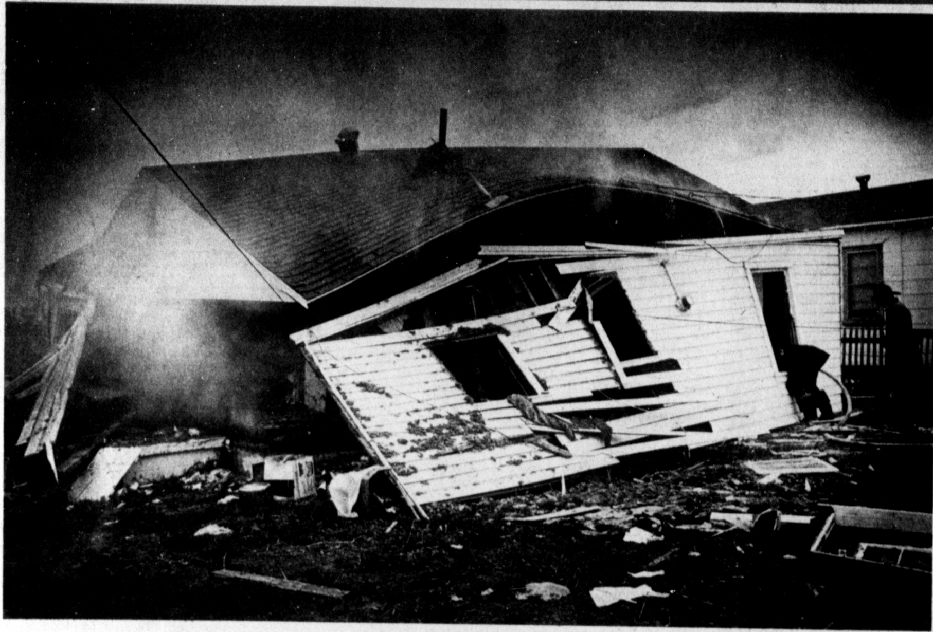
Collapsing walls and a sagging roof are all that's left of a house at 1604 S. Loraine St. following an early morning explosion today. Matt and Janet Wells and their 18-month-old
