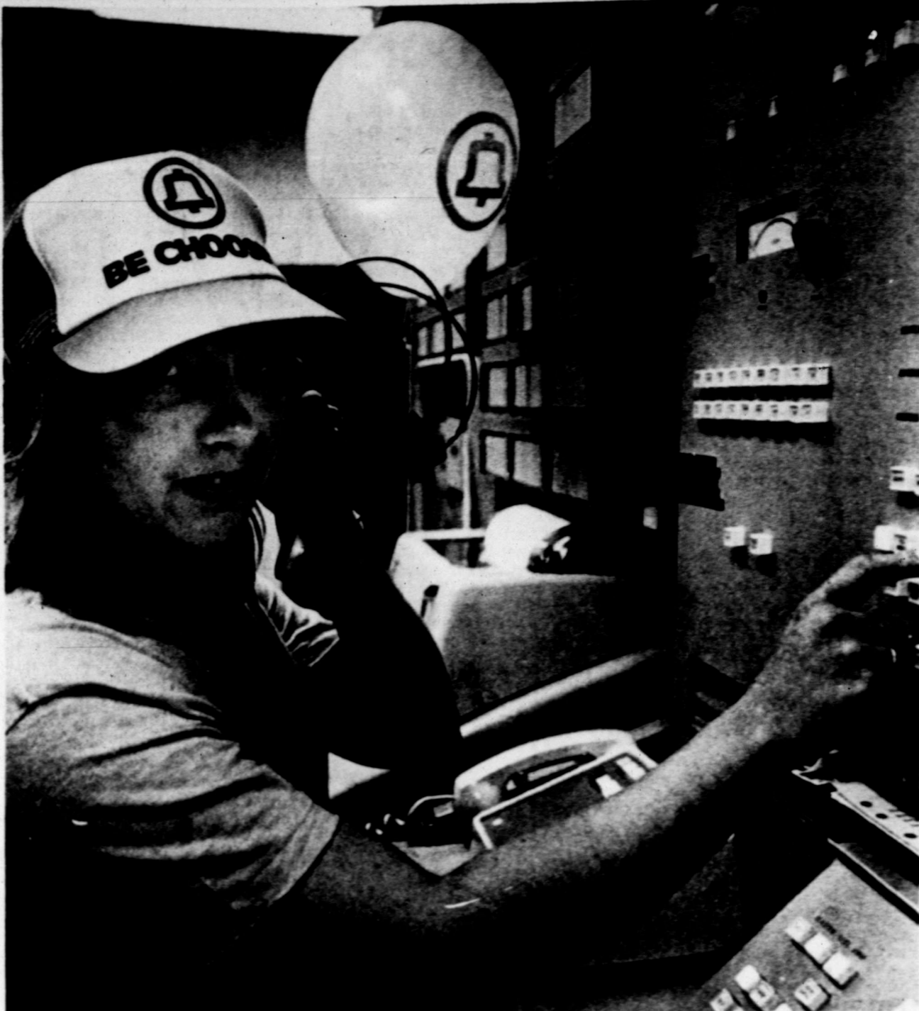
Tish Ford, Electronic Switching System (ESS) technician for Southwestern Bell Telephone monitors Southwestern Bell's new ESS equipment. Bell introduced the second Electronic Switching System
