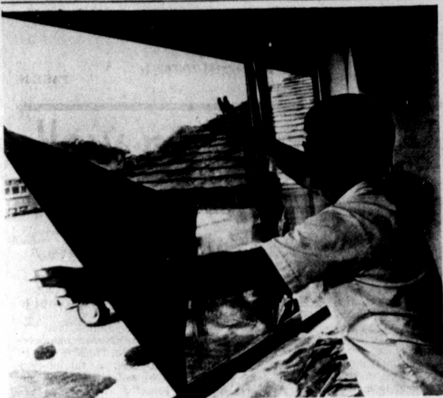
"Scotchint" sun control film by 3M is shown being professionally installed on residential windows. Beauty thus achieved would be reason enough for this installation, but reflection of up to 75 percent of the heat of the summer sun and up to 20 percent reduction of heat loss in winter are compelling reasons for having these benefits for your own home or offices. Call 697-2266 or come by 3M Business Products, West Highway 80.
