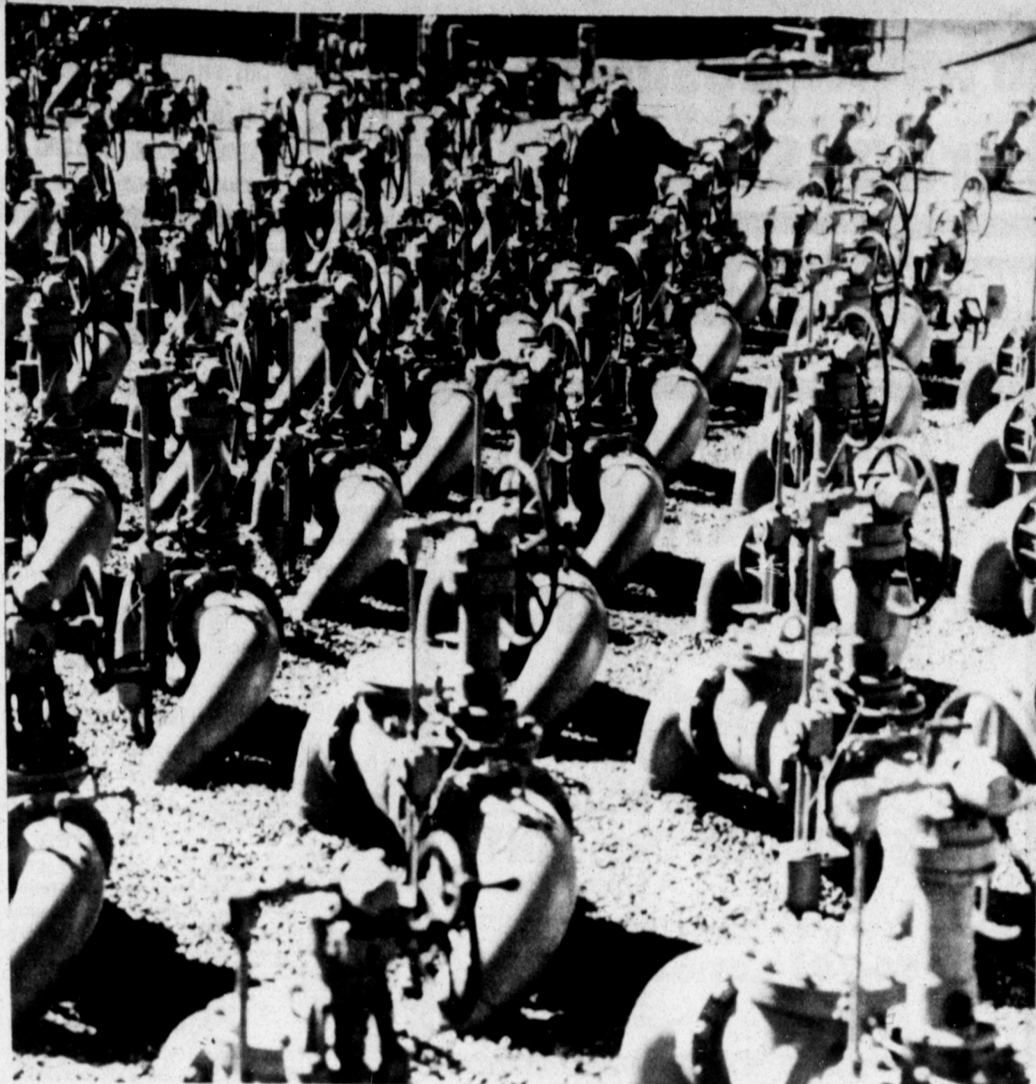
An unidentified technician examines some of the more than 100 shutoff valves grouped at a Long Beach, California, central gathering station. Each bank of valves represents a different petroleum product or refiner. Major oil
