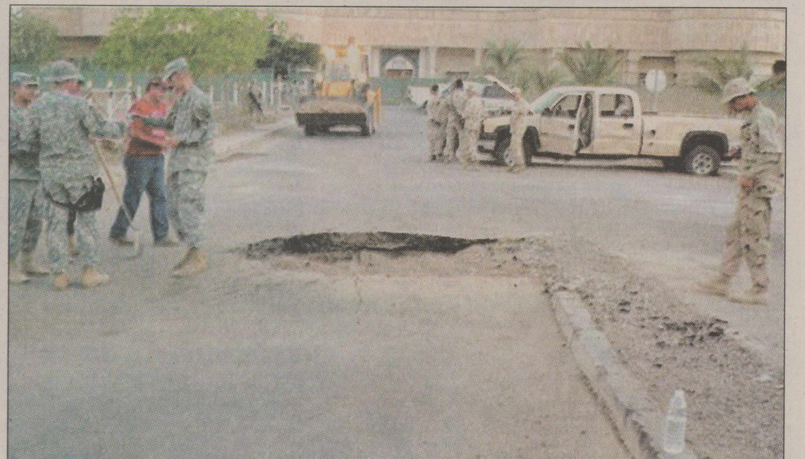
COURTESY PHOTO/Capt. Gary Jones An example of damage done to a road after being hit by indirect fire — one part of Capt. Gary Jones' daily life.
