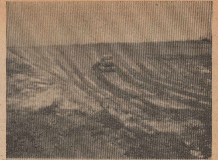
Pond being constructed on the Johnny Burson Ranch. The pond will furnish livestock water and better grazing distribution.
