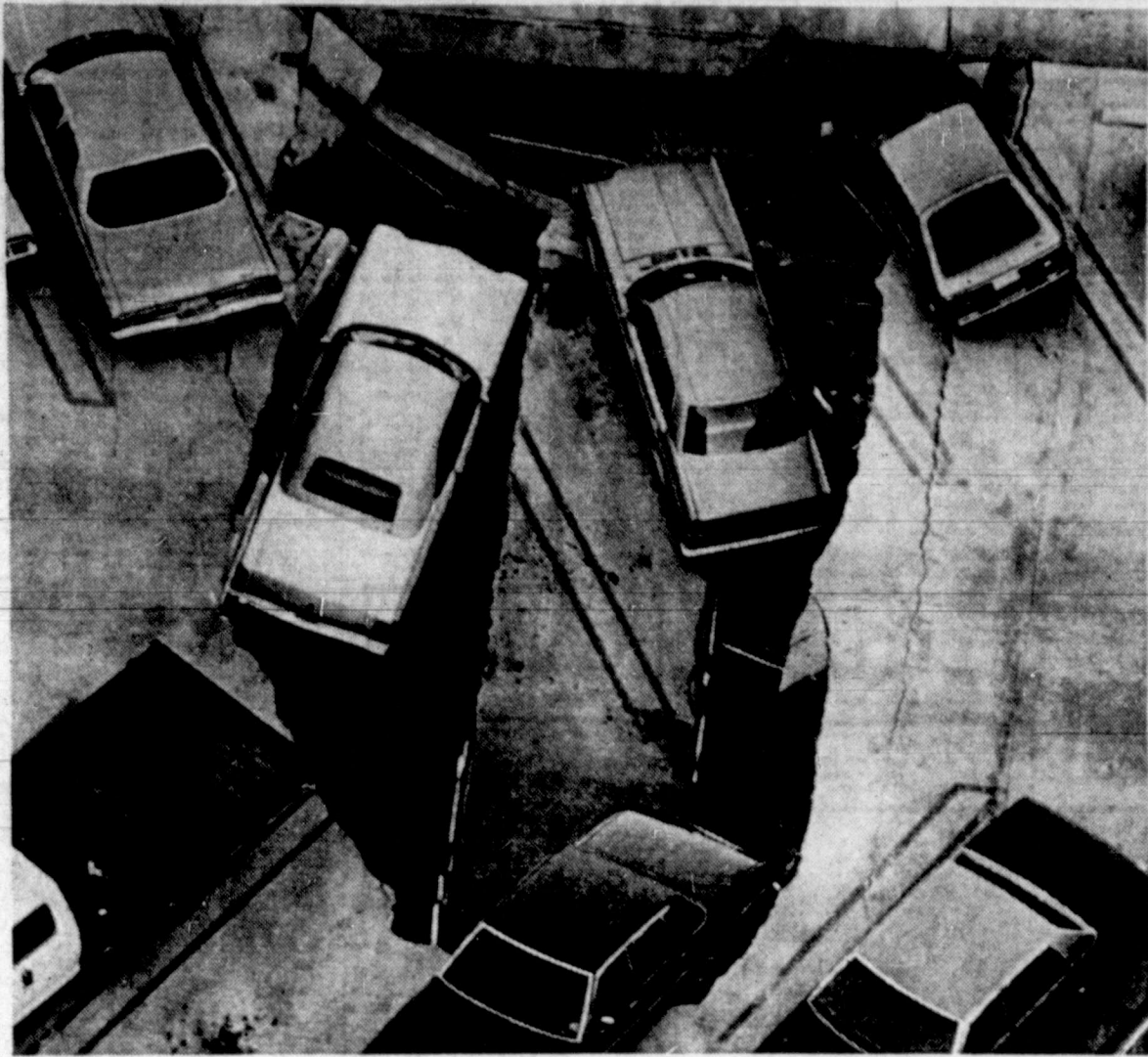
PERILOUS PARKING — A 24-foot beam apparently gave way in the downtown Oklahoma City Oil Center parking garage early Monday. Authorities said there were no injuries, but about a dozen autos were damaged when the top level of the two-tier garage partially collapsed. (AP Laserphoto)
