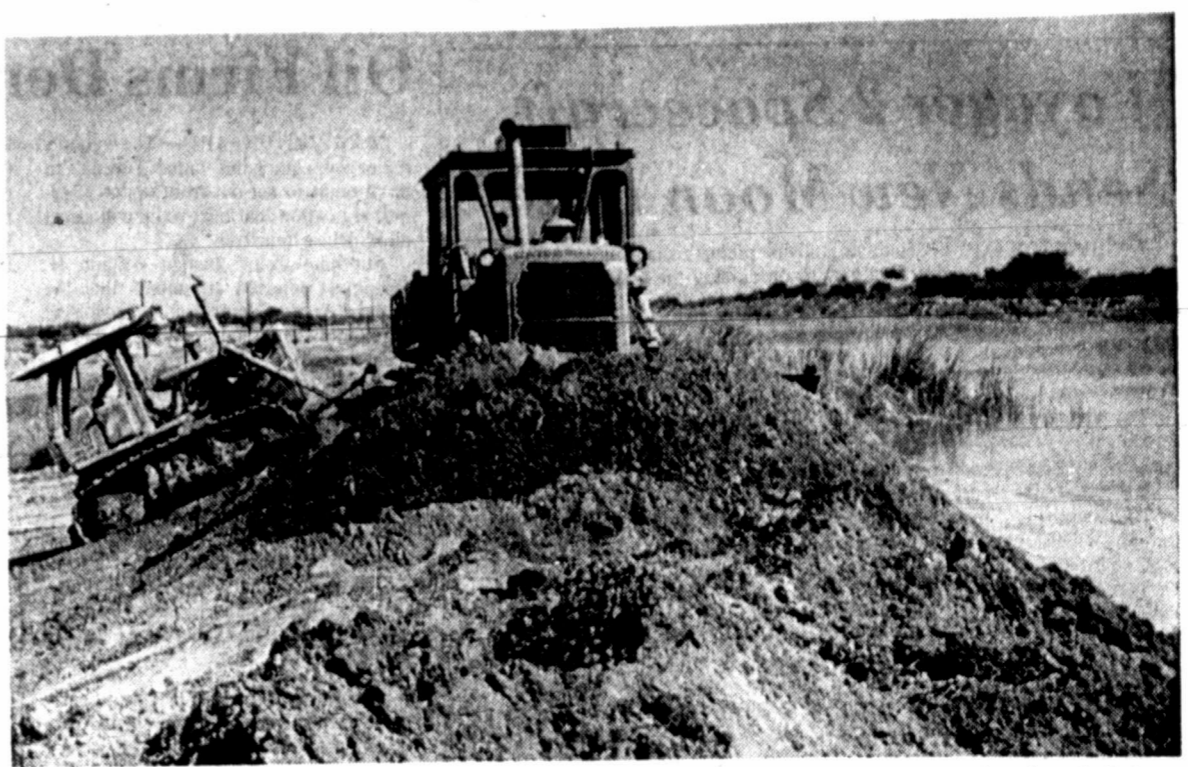
REBUILDING THE CANAL — Bulldozers move earth Tuesday as they rebuild the All-American Canal 16 miles east of Calexico, Calif. The 80-mile canal, which was heavily damaged by an earthquake that struck southern California Monday afternoon, feeds water to a 5,000-mile complex of canals that are used to water the crops grown in the Imperial Valley. Several buildings were damaged in Calexico and elsewhere in southern California. (AP Laserphoto)
