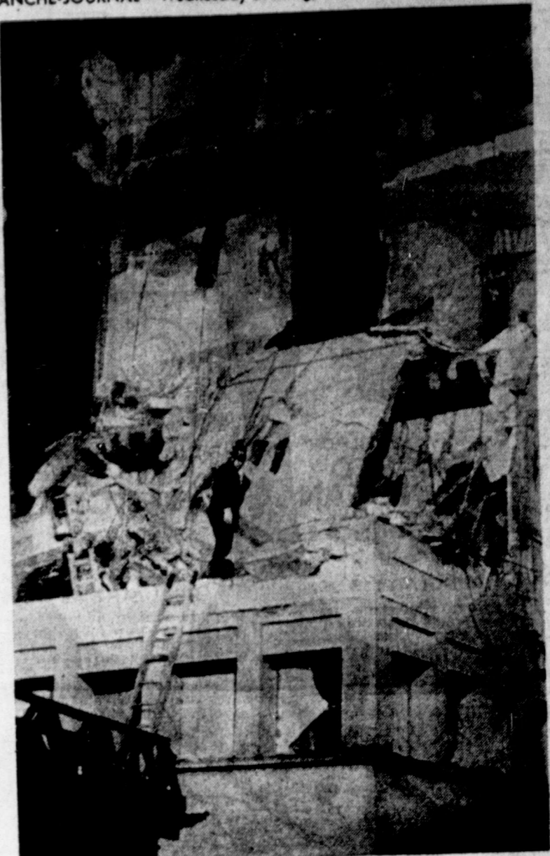
SEARCHING HOSPITAL DEBRIS — Authorities search through the rubble of a demolished wing of the city hospital in Parma, Italy, Tuesday after a gas explosion ripped the building. At least seven persons were killed with the chance the death toll will rise higher as rescue teams continue their search for 23 persons believed trapped beneath the wreckage. (AP Laserphoto)
